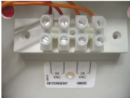
Terminal block before connecting power wires
